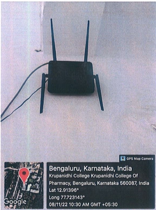
2 nd FLOOR Wi-Fi
