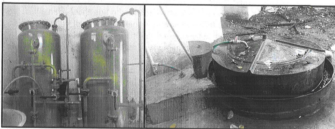
Biogas plant set up in the KCP, Bengaluru, Karnataka.
